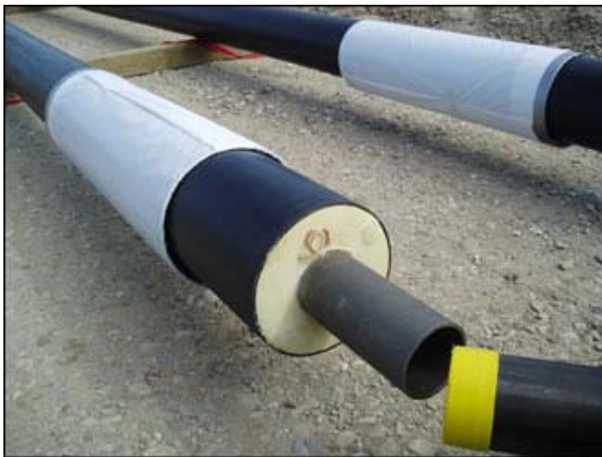
Pipes for district heating with hot water.
